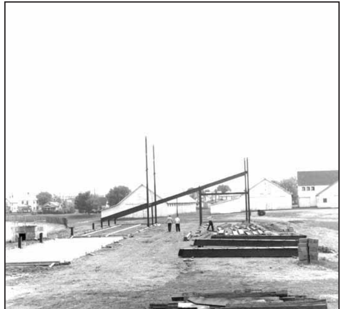
THE NEW GRANDSTAND BEING BUILT AT THE COSHOCTON COUNTY FAIRGROUNDS SUMMER OF 1954.
